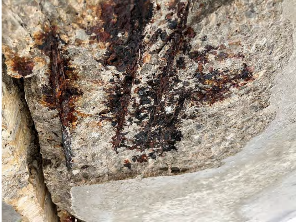
Photo No. 3 2/16/2022 Looking at 4 prestressed strands on south exterior beam 1/3 span
