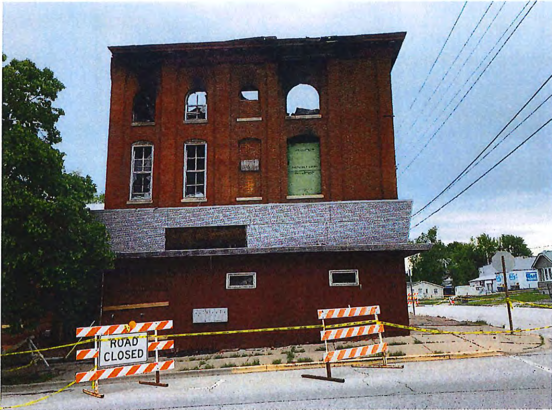
649 State Street Damage from Fire on May 18, 2022 Photos taken May 24, 2022
