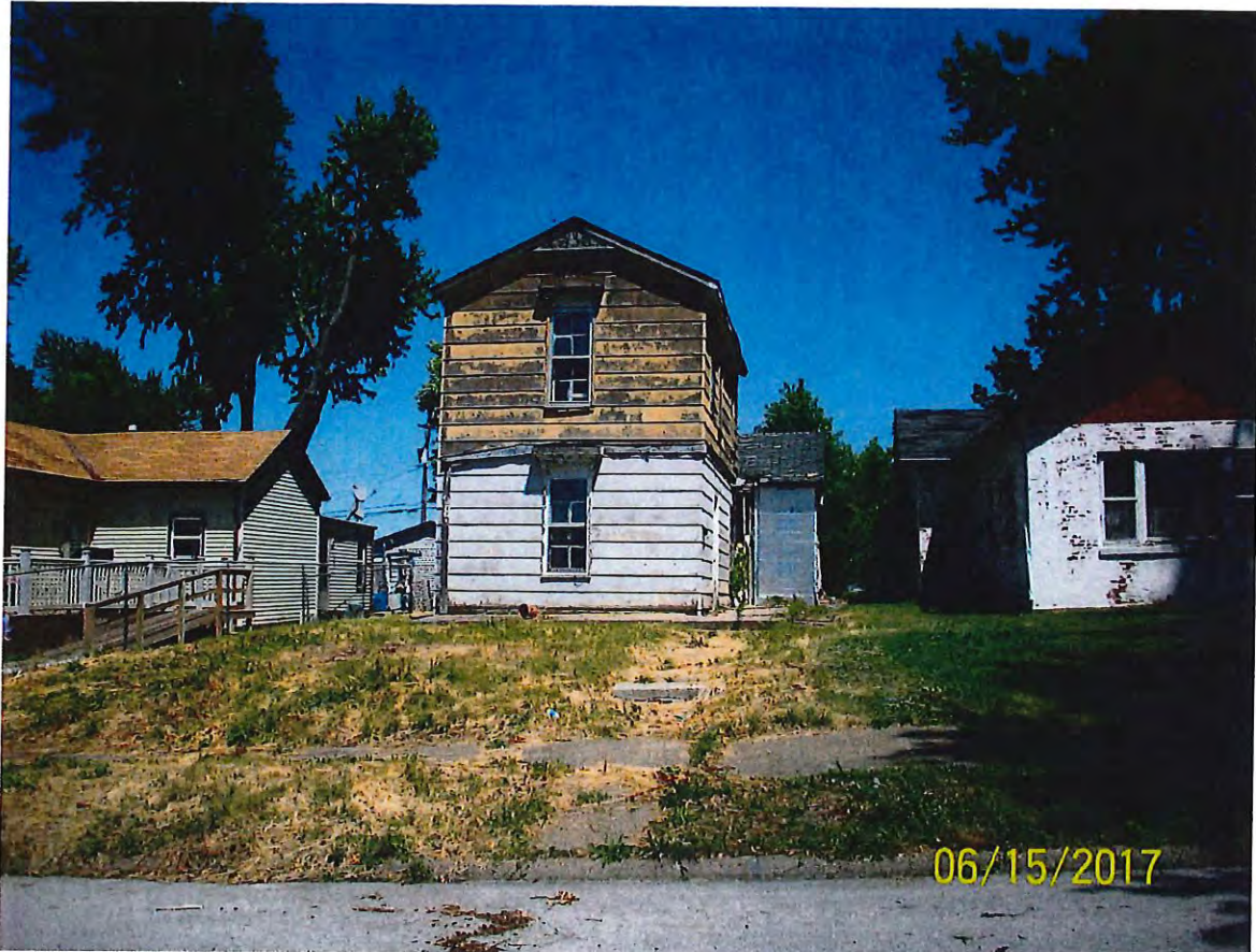
1422 N. 9th St. / As observed on 6-15-2017
