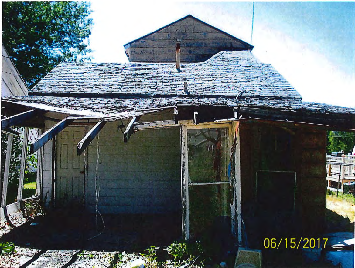
1422 N. 9th St. / As observed on 6-15-2017
